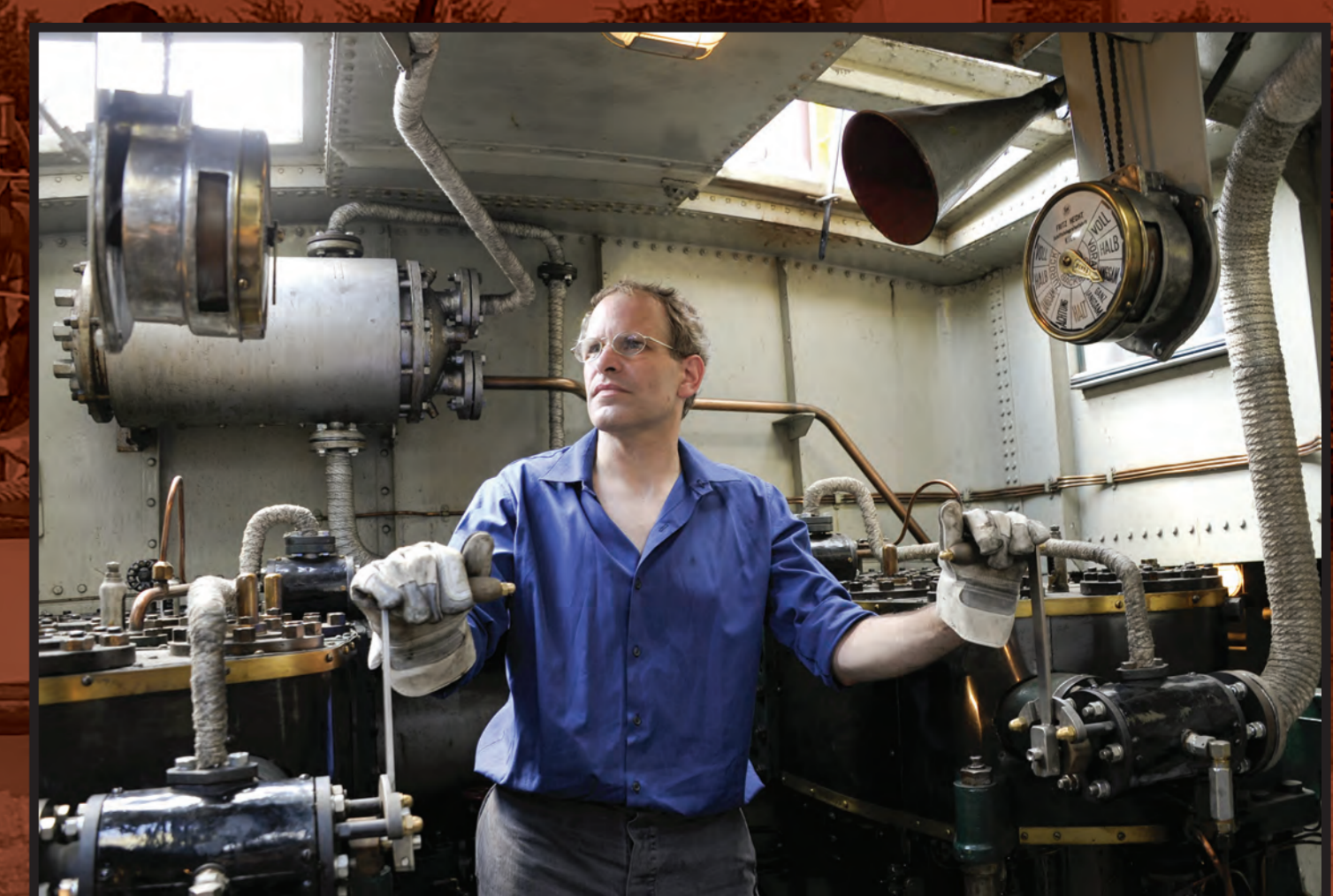
The operator in the engine room, 2012
